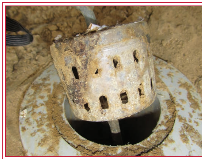
Empty in-ground canister following Coptotermes feeding.
